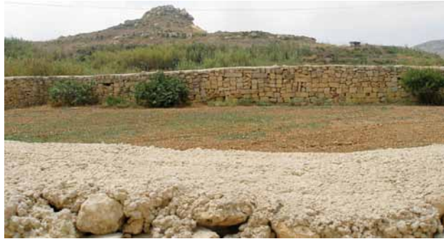
Figure 9: A layer of concrete at the top of a wall to quickly repair it.
