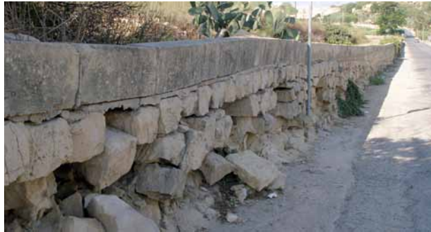
Figure 10: A repaired wall with its older layers falling away.
