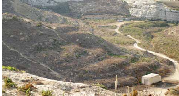
Figure 3: Terrace walls that have gone unmaintained allowing the hill to erode back to its natural state.
