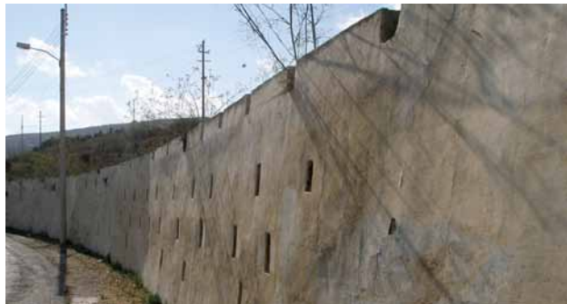
Figure 8: Drainage pipes in a modern wall.
