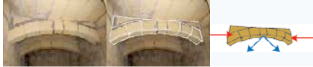
Figure 22: Detail of an arch that functions as a bearing construction for the roof.
