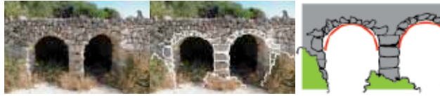
Figure 21: Arch from smaller stones without a keystone in the centre has poorer construction properties.
